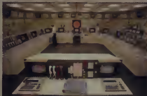
Hope Creek power plant control room simulator.
